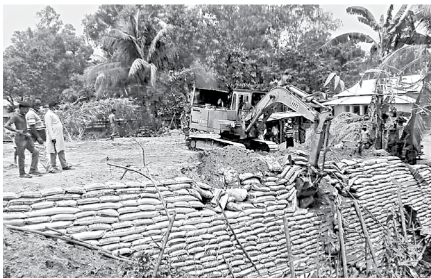
A mobile court in a drive recovered this portion of an important canal, illegally occupied by some local influential people. The photo was taken from Bhuanpara area in Tangail's Gopalpur upazila a few days ago.
