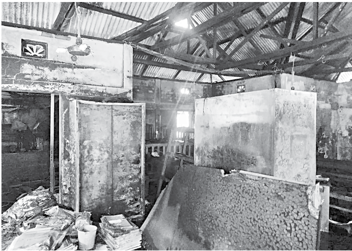
At least five semi-pucca rooms, including the UP chairman's office, union health and family welfare centre and village court room, furniture and important documents were completely burnt to ashes when a fire broke out at Dakkhinbhat Uttar Union Parishad office in Moulvibazar's Barlekha upazila yesterday morning.
