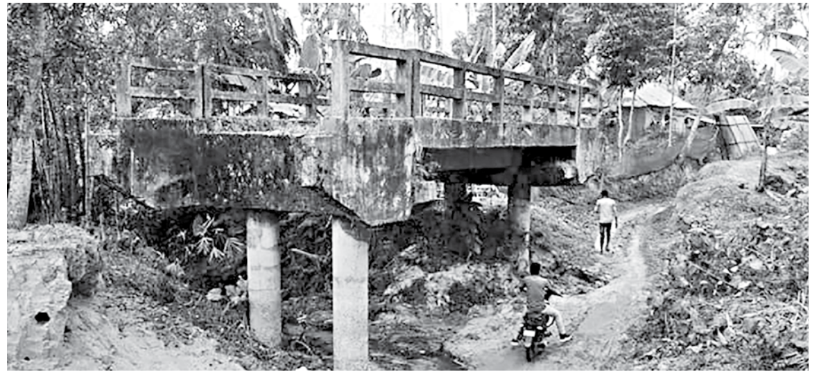
A motorbike rider negotiates the rough dry creek below the flawed bridge, in Dilbaragar village of Moulvibazar's Srimangal upazila, which lies without approach roads for 21 years.
