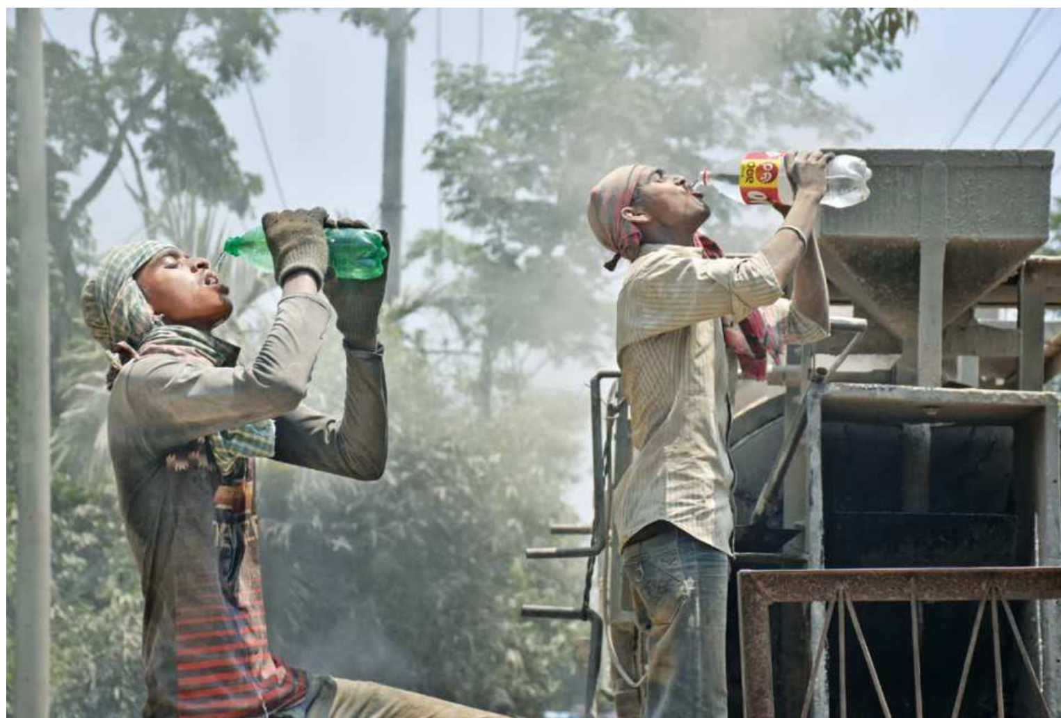
On road construction duty in the burning heat of yesterday's noon, two workers take a break from mixing stone with bitumen and to rehydrate themselves. A heat wave is sweeping the country, and those who have to do hard physical labour -- especially outdoors -- are taking the heat, quite literally. This photo was taken from Barishal city's Kaladema area.
