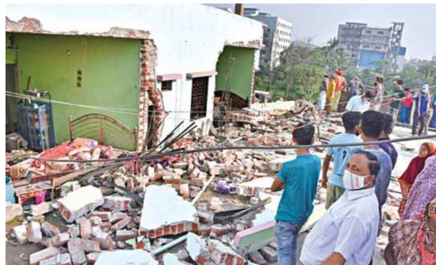
A portion of a wall of the building collapsed due to the gas explosion. PHOTO: STAR
