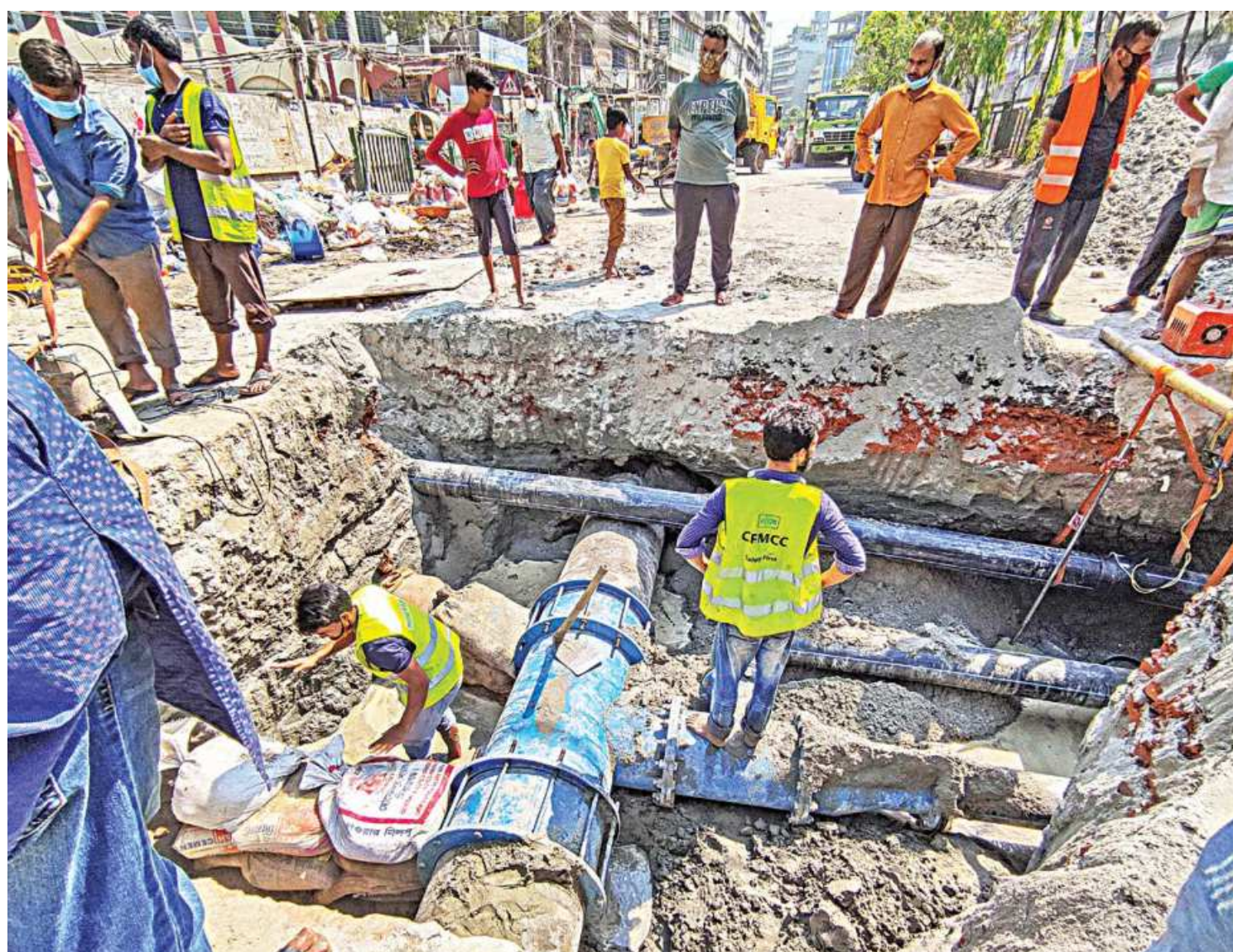
To improve the water supply in Old Dhaka, Dhaka Wasa authorities are installing a 250-inch pipeline in the area. Though this kind of operations are usually a nuisance for commuters, this one is causing less of a disturbance during the lockdown. This photo was taken from North South Road yesterday.
