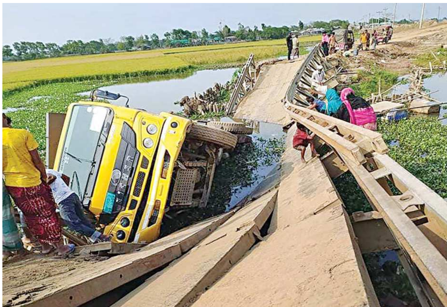
A Bailey bridge on Netrokona-Kamalkanda road in Kamalkanda upazila of Netrokona collapsed yesterday when an overloaded truck was crossing it. It was constructed around two years ago as a diversion bridge.
