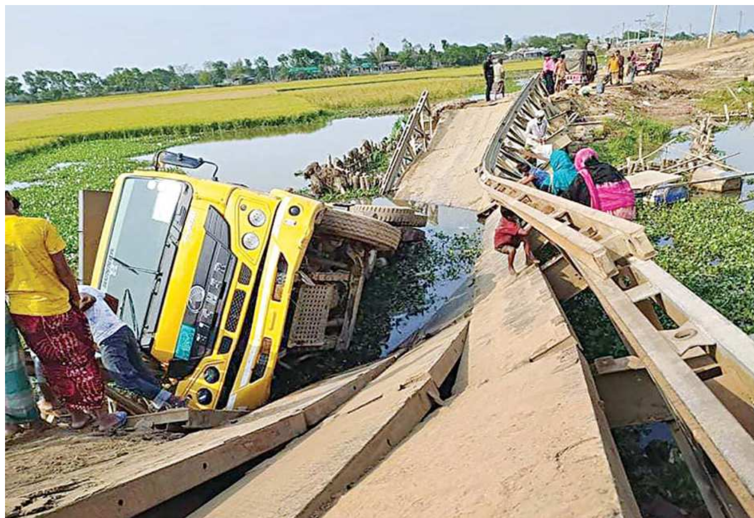
A Bailey bridge on Netrokona-Kamalkanda road in Kamalkanda upazila of Netrokona collapsed yesterday when an overloaded truck was crossing it. It was constructed around two years ago as a diversion bridge.
