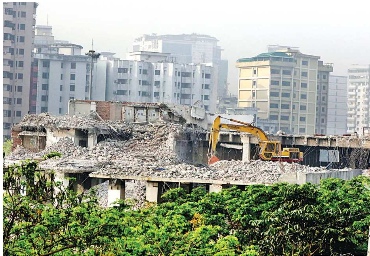
This photo taken recently shows just one floor of the once multi-storey BGMEA Building still standing in the capital's Hatirjheel area. Rajdhani Unnayan Kartripakkha started knocking down the building in January last year in accordance with a High Court ruling.
