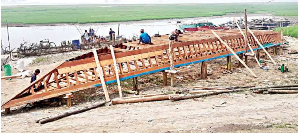
Workers build a boat along the Jamuna river in Tangail's Bhuiyanpur upazila. Boat becomes the only means of communication in some remote char areas of Tangail, Sirajganj and Jamalpur districts during the rainy season. The photo was taken recently.
