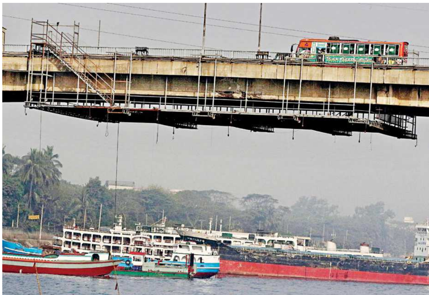
Scaffoldings have been set up under the First Bangladesh-China Friendship Bridge, also known as Postogola Bridge, for its repairs. The bridge was damaged by a BIWTA salvage ship that did not lower its crane while going under it in June last year. This photo was taken on Friday.
