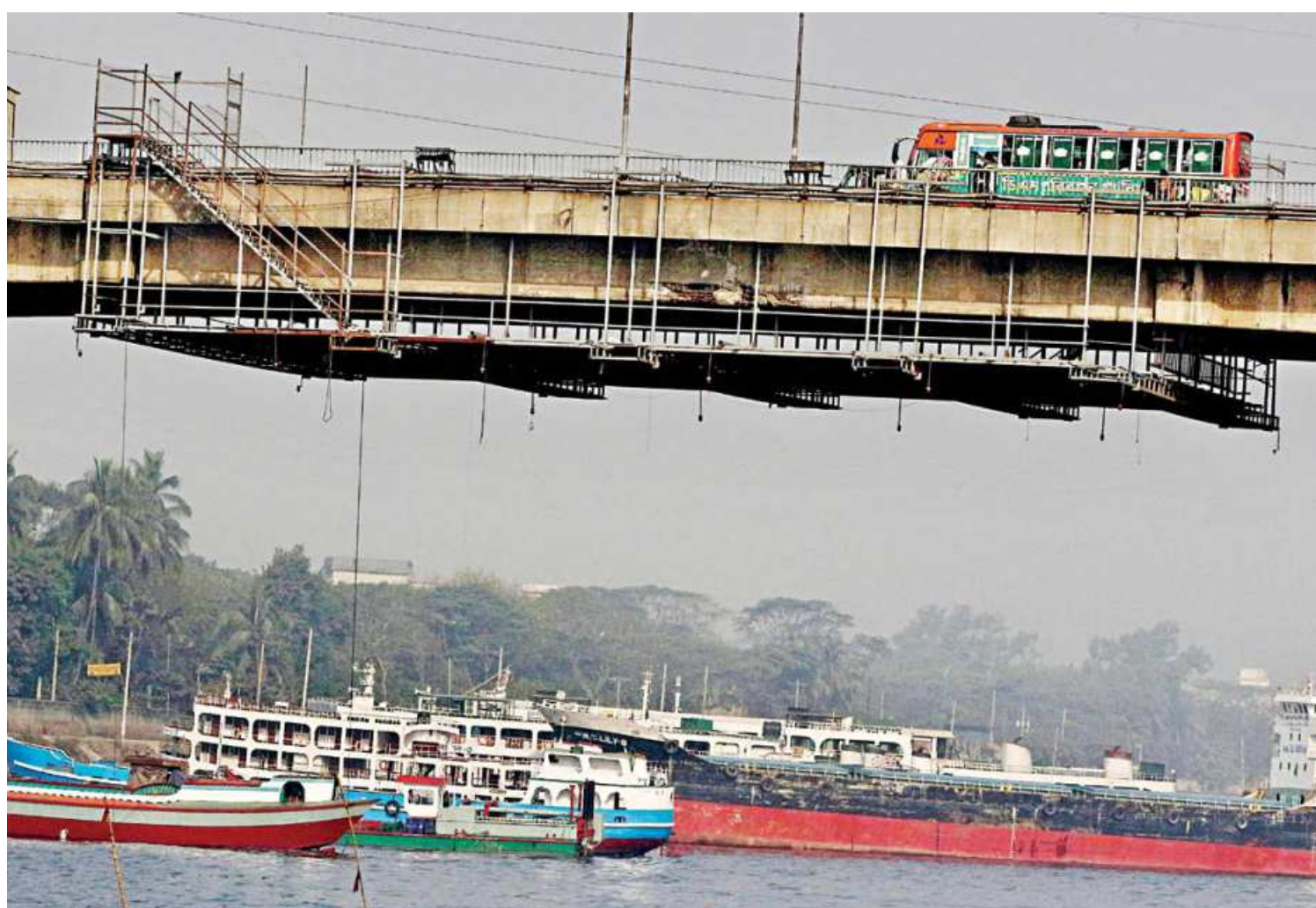
Scaffoldings have been set up under the First Bangladesh-China Friendship Bridge, also known as Postogola Bridge, for its repairs. The bridge was damaged by a BIWTA salvage ship that did not lower its crane while going under it in June last year. This photo was taken on Friday.
