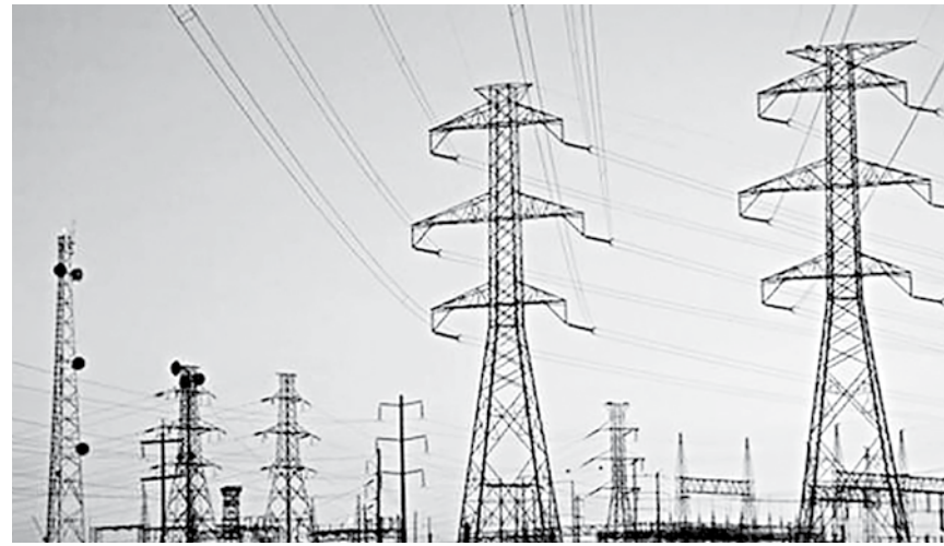
The government invested roughly USD 15 billion in electricity generation against only USD 1.5 billion in transmission and USD 2.6 billion in distribution since 2009.
