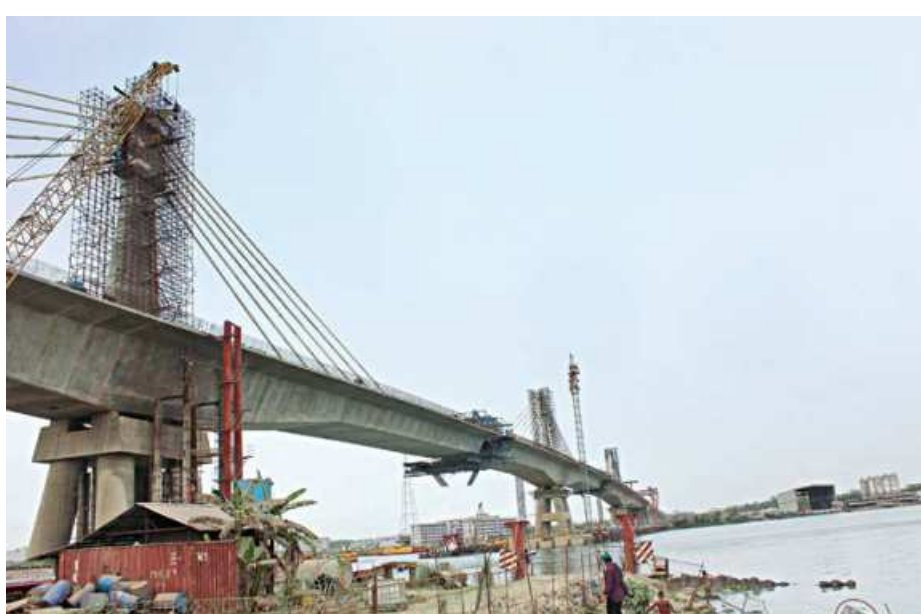
About 90 per cent of the main bridge is complete while the construction of ancillary structures is ongoing.
