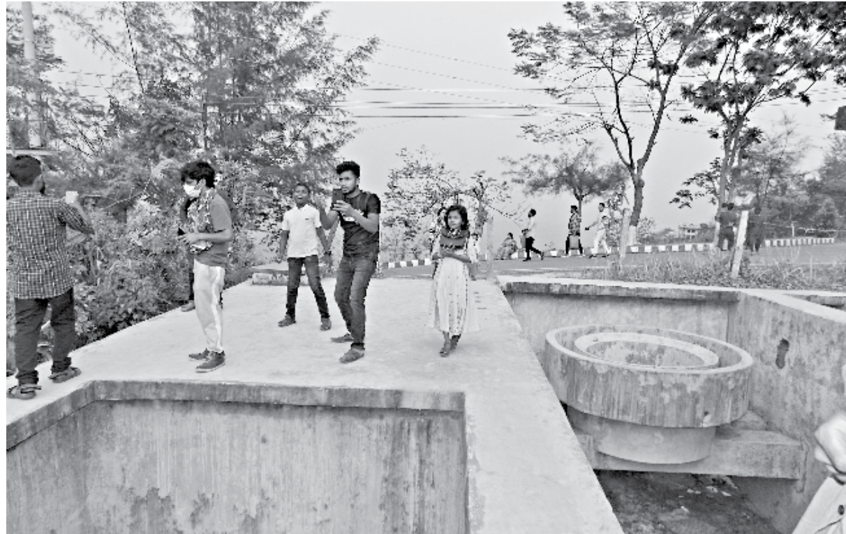
Without any boundary fence around, the large open pits of the incomplete water supply facility, for Neelachal tourist spot in Bandarban, can turn fatal for any of the curious passersby any moment. The photo was taken recently.
