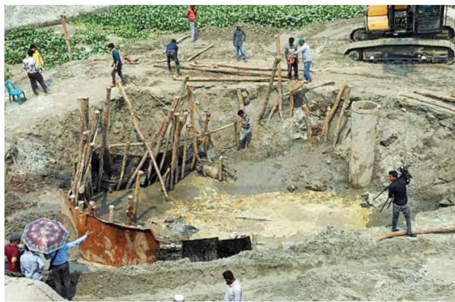
Titas gas authorities repairing a gas pipe damaged during the construction work of Salehpur Bridge on Dhaka-Aricha highway. The bridge is being constructed by the Roads and Highways Department.
