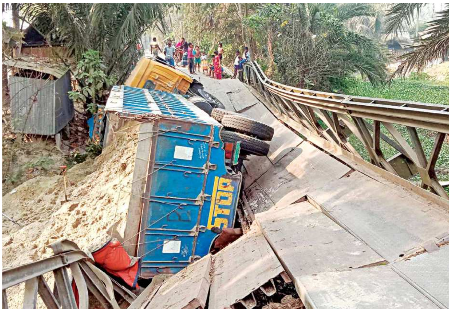
A sand-laden truck causes a Bailey bridge on the Mara Chitra river in Mollahat upazila of Bagerhat to collapse early yesterday. Bagerhat Roads and Highways Department executive engineer said there were 10 such bridges on that stretch of road and none of them could withstand so much load.
