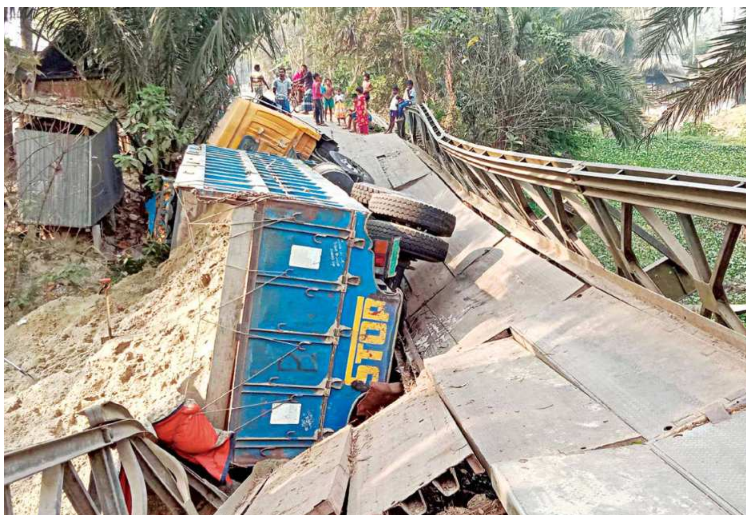
A heavily loaded sand laden truck causes a Bailey bridge on the Mara Chitra River in Mollahat upazila of Bagerhat to collapse early yesterday morning. Bagerhat Roads and Highways Department executive engineer said there were 10 such bridges on that stretch of road and none of them could withstand so much load.
