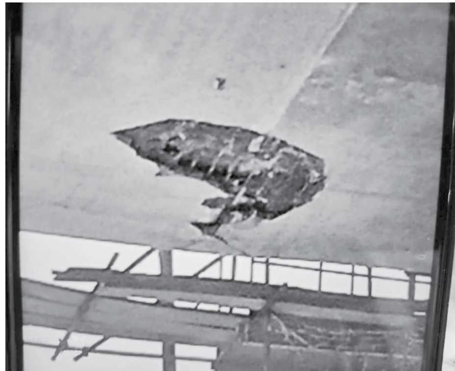
A small section of concrete surface -- about 2 feet long and 1.5 feet wide -- appears to have fallen off near the second pier on the southern end of Payra bridge, currently under construction in Patuakhali's Lebukhali area.
