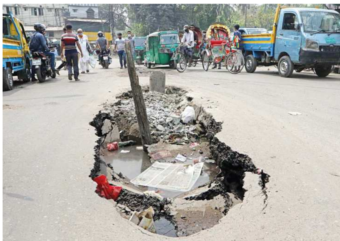
A large hole was created in the middle of the road in the capital's Bangshal about two weeks ago, allegedly due to development work carried out by Dhaka Wasa. However, there has been no initiative to fix the road, and the stick that locals put there to warn oncoming vehicles does little to prevent accidents from occurring every now and then. The photo was taken yesterday.
