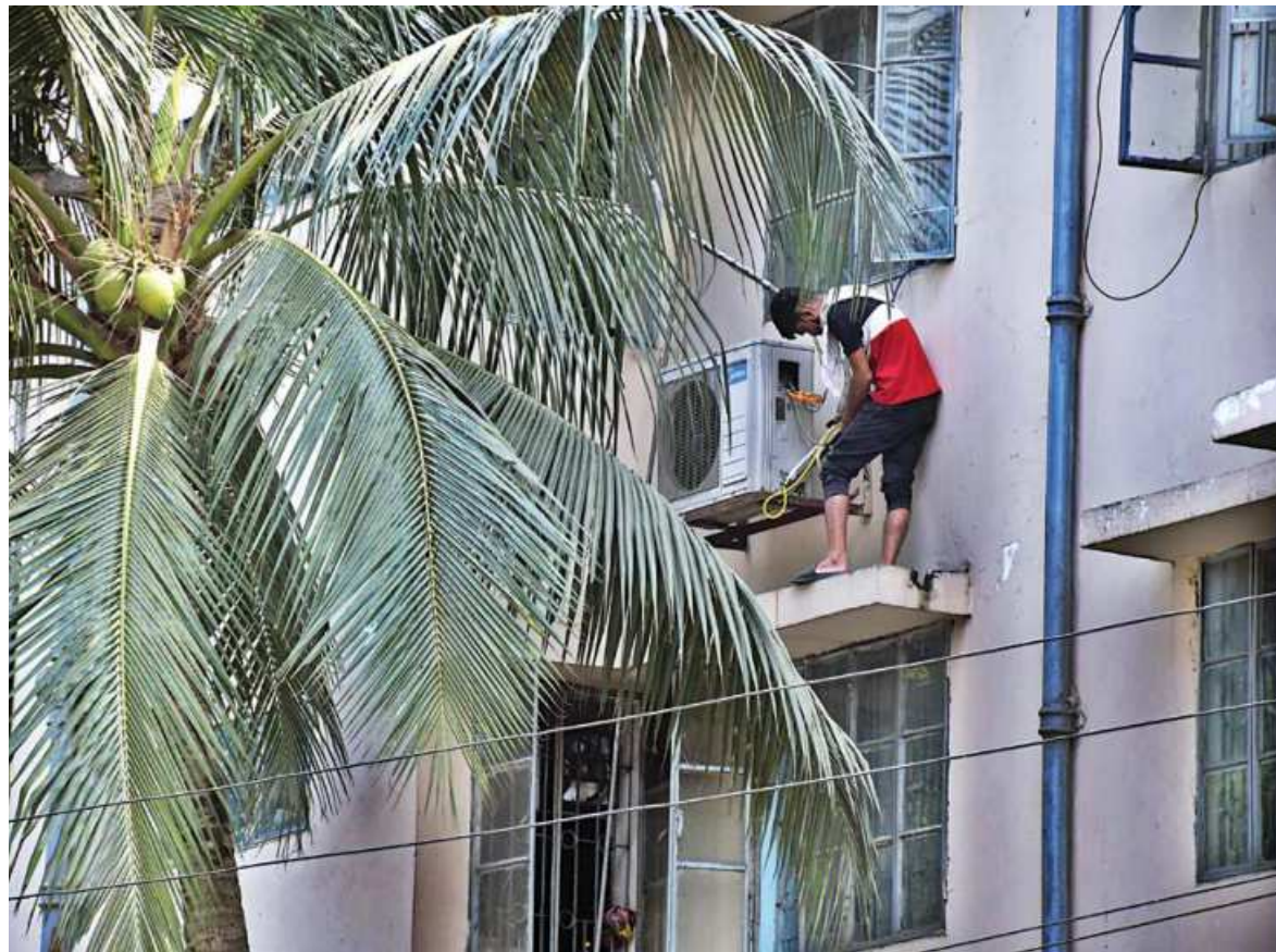
An air-conditioner mechanic stands on a narrow window ledge to fix the appliance, with no safety harness. As summer is in full gear, such mechanics can be seen in precarious positions in the coming days, neglecting safety equipment. This photo was taken yesterday from Dhaka University area.
