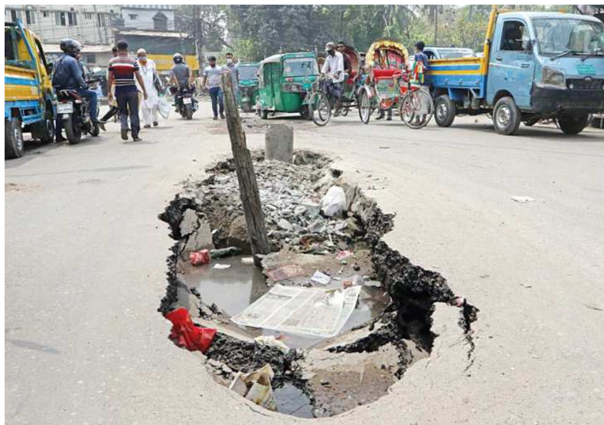
A large hole was created in the middle of the road in the capital's Bangshal about two weeks ago, allegedly due to development work carried out by Dhaka Wasa. However, there has been no initiative to fix the road, and the stick that locals put there to warn oncoming vehicles does little to prevent accidents from occurring every now and then. The photo was taken yesterday.
