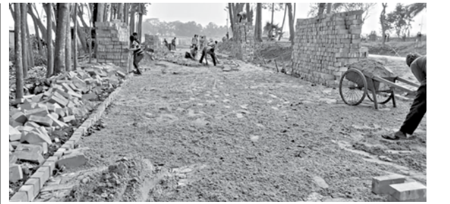
A road being constructed ahead of Narendra Modi's visit to Orakandi Thakur Bari Temple, below, in Gopalganj's Kashiani upazila.
