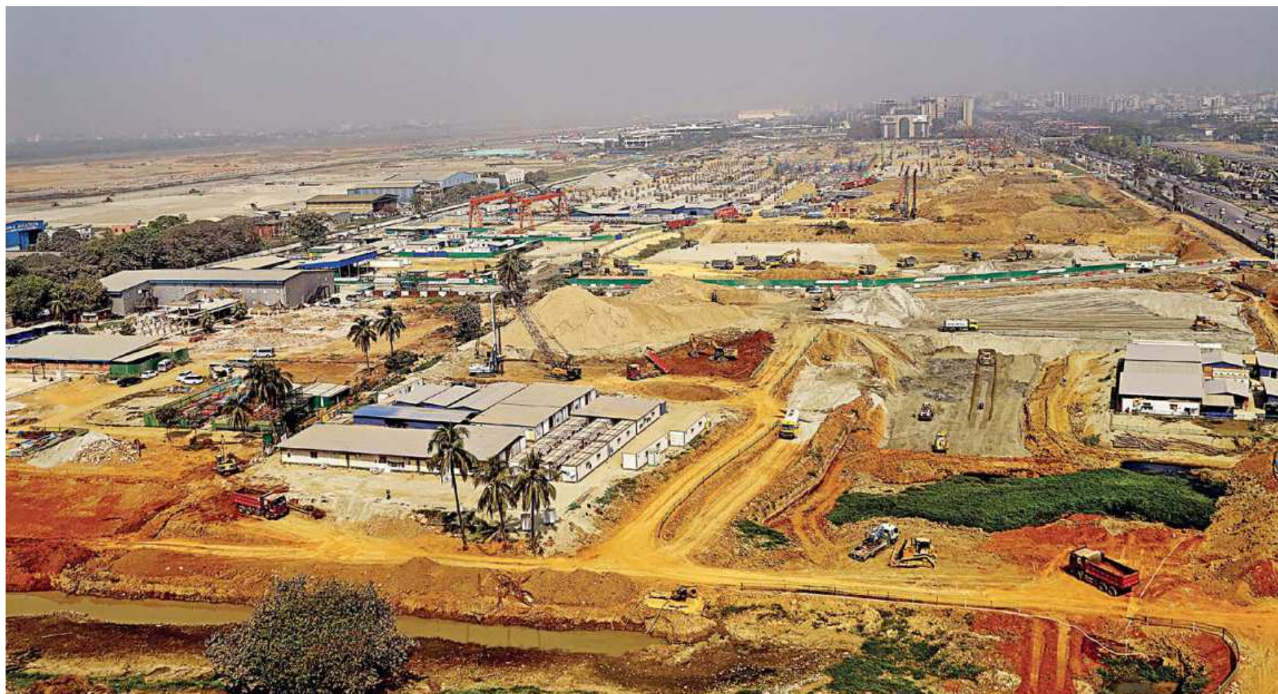
The under-construction third terminal of Hazrat Shahjalal International Airport. The Tk 21,399 crore project is funded by Jica and the Bangladesh government. Mitsubishi and Fujita of Japan and Samsung of Korea are expected to complete the work by June, 2023. The photo was taken a couple of days ago.
