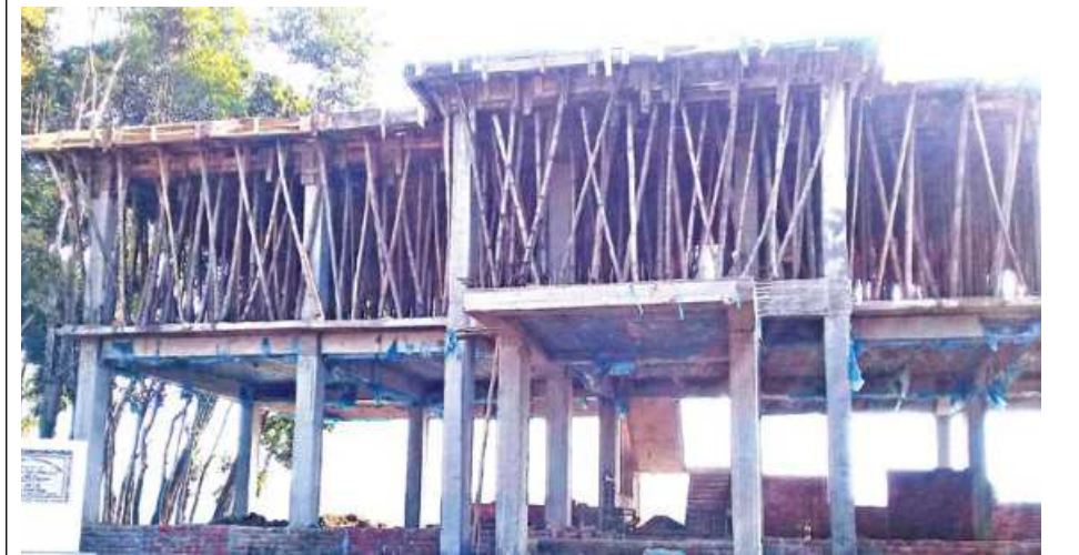
The under-construction building of Barni Union Health and Family Welfare Centre in Moulvibazar's Barlekha upazila. PHOTO: STAR
