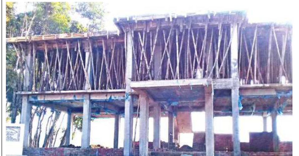
The under-construction building of Barni Union Health and Family Welfare Centre in Moulvibazar's Barlekha upazila.
