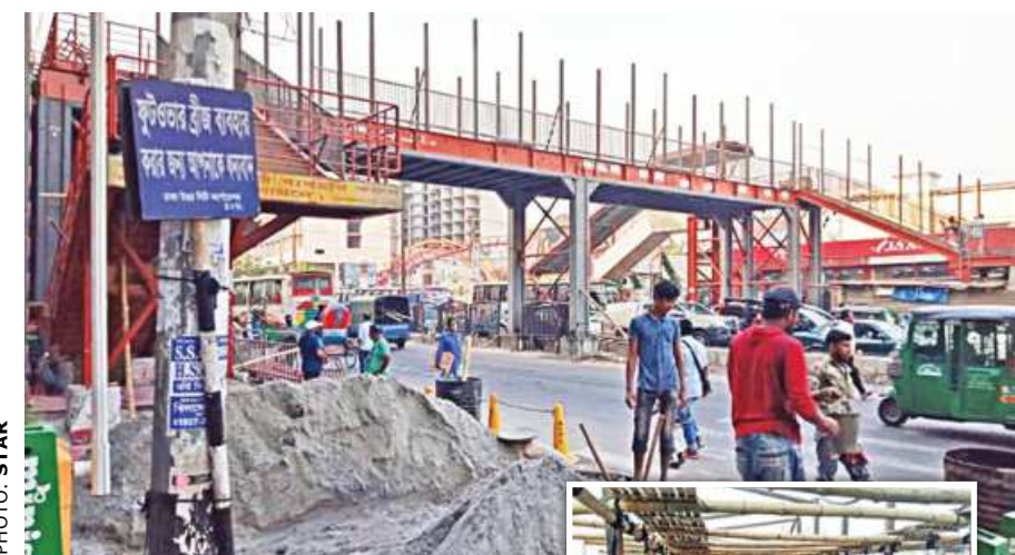
A sign saying "Thank you for using the footbridge" stands in irony on Pragati Sarani in the capital, as work continues on the structure. Inset, workers were recently seen replacing the railings of the bridge.
