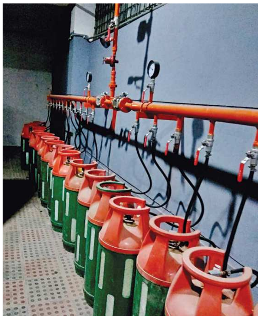
Gas cylinders lined up on the ground floor of a multi-storey apartment building in Ulon area of Rampura in the capital. The cylinders are kept there and connected to the kitchens upstairs using pipes as the apartment residents fear that the cylinders might explode. The photo was taken yesterday.
