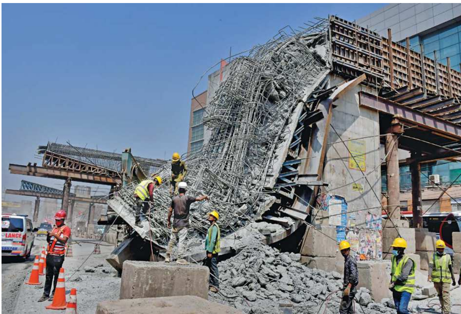
Construction workers inspecting a collapsed pier cap of the Bus Rapid Transit project in front of the Polwel Carnation Shopping Centre in Uttara. The pier cap had collapsed early yesterday. In a separate incident hours later, a portion of a launching girder of the same project collapsed near Dhaka airport around 10:30am, leaving six workers, including three Chinese nationals, injured.
