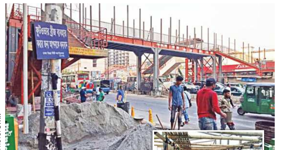
A sign saying "Thank you for using the footbridge" stands in irony on Pragati Sarani in the capital, as work continues on the structure. Inset, workers were recently seen replacing the railings of the bridge.
