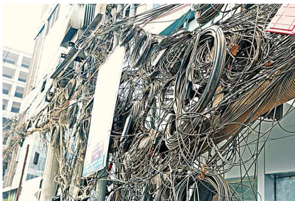
Despite HC rulings and repeated warnings, cables and wires hung from electric polls keep cluttering up Dhaka residents' line of sight. But beyond just an eyesore, they also pose the danger of short circuits and explosions. This photo was taken from Karwan Bazar area yesterday.
