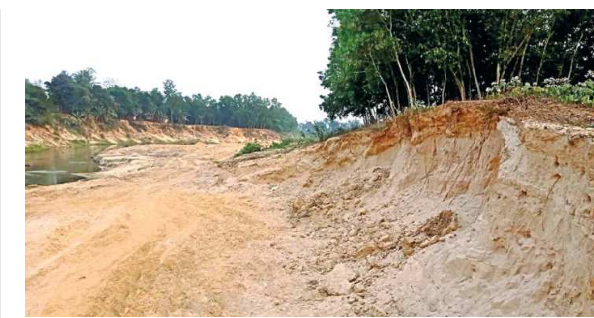
Wounds on the bank of the Halda river as sand and earth litters wreaked havoc on the river in Fatikchhari upazila.
