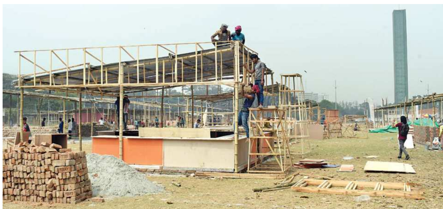
Construction of stalls and pavilions is in full swing at the capital's Suhrawardy Udyan, ahead of Ekushey book fair. From March 18, this open field will be full of avid readers zigzagging across all the stalls around them and contemplating which books to buy. This photo was taken yesterday.
