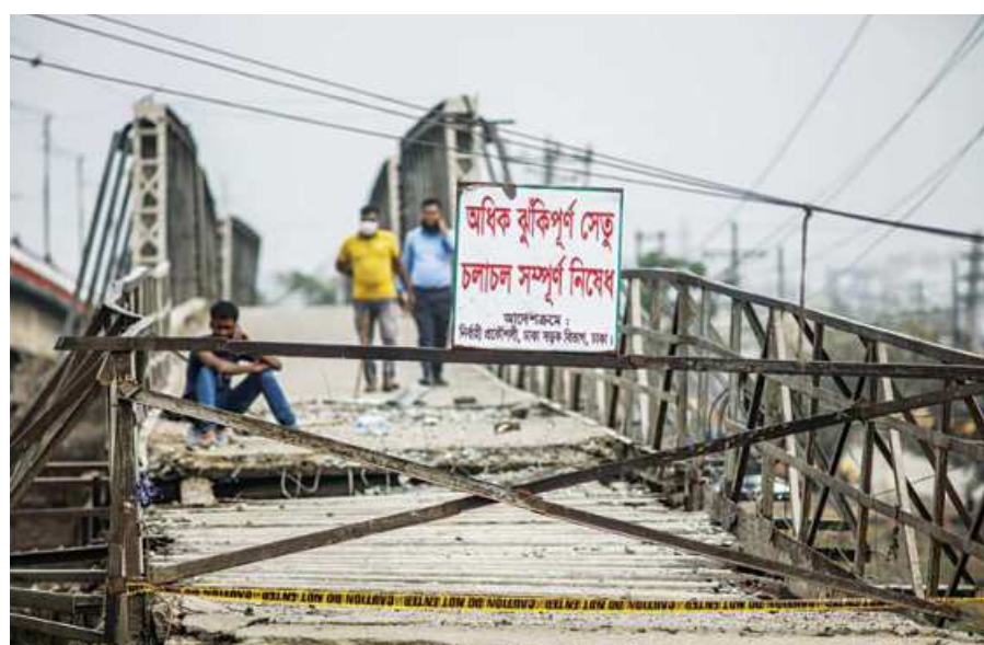
Two people walking on a bridge in Aminbazar on the Dhaka-Aricha highway yesterday. As the sign says, the bridge has been closed to the public because it is risky and a part of it has even collapsed, but people use the structure despite the risks.
