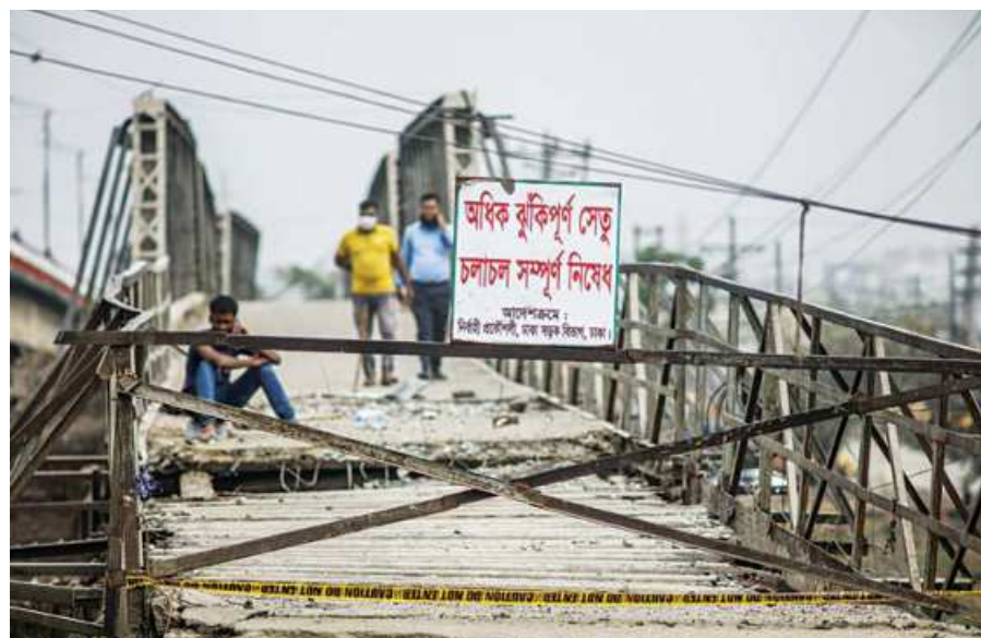
Two people walking on a bridge in Aminbazar on the Dhaka-Aricha highway yesterday. As the sign says, the bridge has been closed to the public because it is risky and a part of it has even collapsed, but people use the structure despite the risks.
