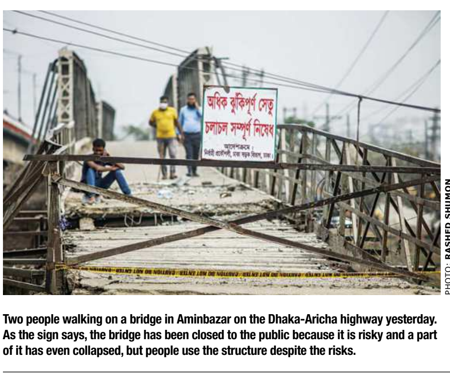
Two people walking on a bridge in Aminbazar on the Dhaka-Aricha highway yesterday. As the sign says, the bridge has been closed to the public because it is risky and a part of it has even collapsed, but people use the structure despite the risks.
