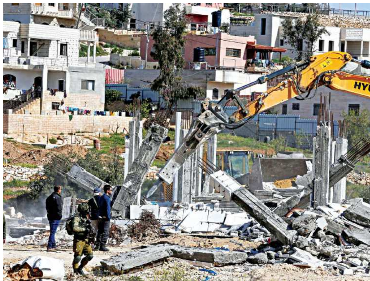
A machinery guarded by Israeli forces demolishes an under-construction Palestinian building, in Bani Naim near Hebron in the Israeli-occupied West Bank yesterday.
