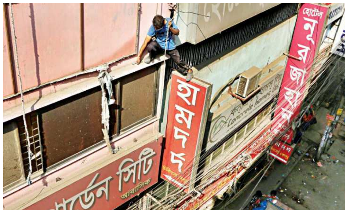
Holding only a piece of rope and equipped no other safety gear, a man works to set up a billboard in the capital's Moghbazar area. He could fall, badly injured himself or even die. The photo was taken yesterday.
