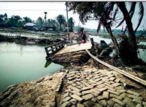
"It is high time we take necessary steps to reconstruct the damaged parts of the embankments, otherwise during the next cyclone the effect will be catastrophic" - Ripon Kumar Mondal, Chairman, Deluti Union, Paikgachha
