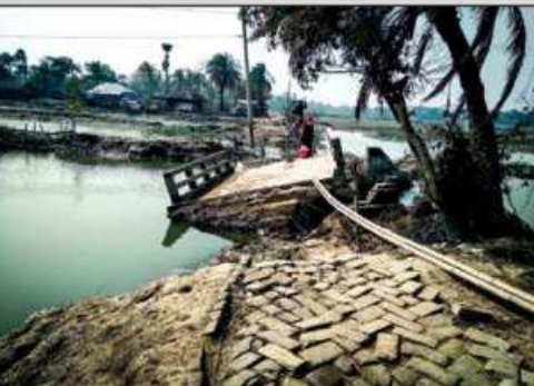
"It is high time we take necessary steps to reconstruct the damaged parts of the embankments, otherwise during the next cyclone the effect will be catastrophic" - Ripon Kumar Mondal, Chairman, Deluti Union, Paikgachha
