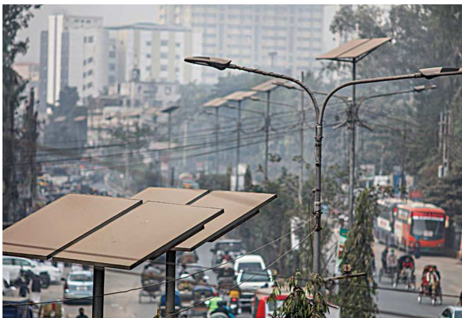
A thick layer of dust on the solar panels that recharge the street lights in Fakirpool area of the capital. If the panels are not cleaned properly at regular intervals, it renders them unable to generate adequate power from the sun.
