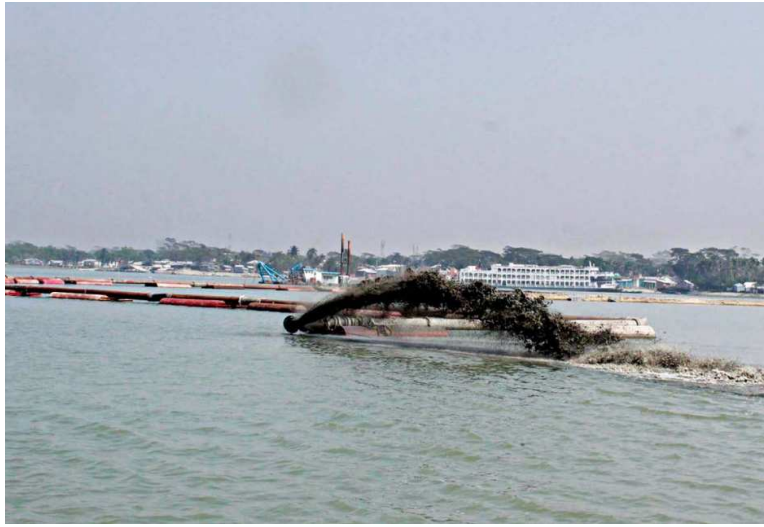
Discharge from a dredger is being dumped straight into the Payra river near Amtali Ferry Terminal in Barguna making the dredging efforts futile as the silt will eventually clog up another part of the river key for water transport. The photo was taken recently.
