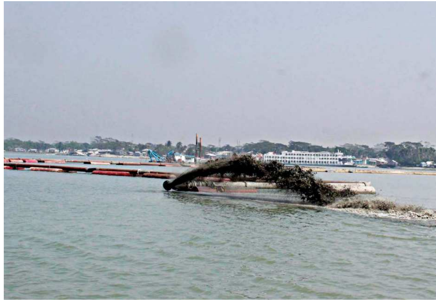
Discharge from a dredger is being dumped straight into the Payra river near Amtali Ferry Terminal in Barguna making the dredging efforts futile as the silt will eventually clog up another part of the river key for water transport. The photo was taken recently.
