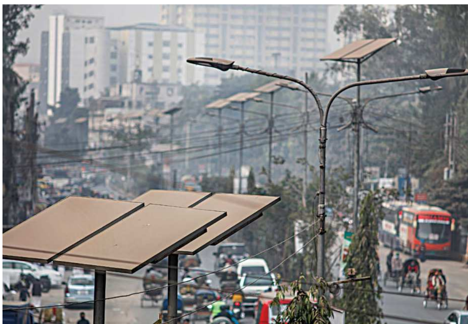
A thick layer of dust on the solar panels that recharge the street lights in Fakirpool area of the capital. If the panels are not cleaned properly at regular intervals, it renders them unable to generate adequate power from the sun.
