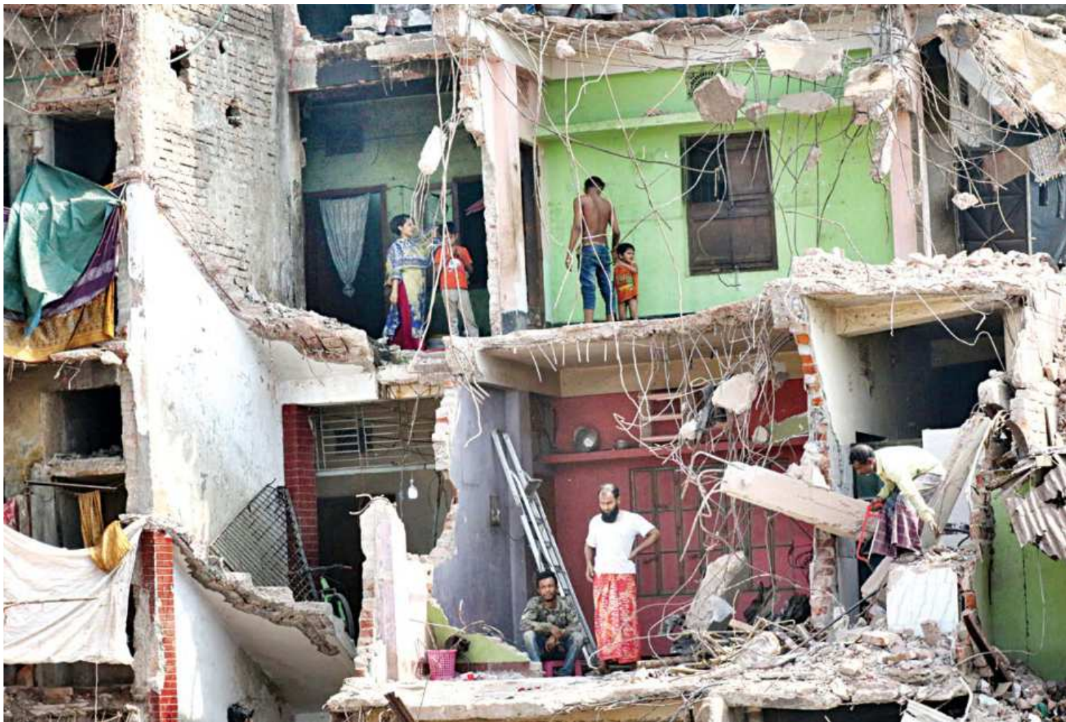
People live in an unsafe three-storey building along the Buriganga in the capital's Lalbagh area. Many buildings in the area were knocked down partially during eviction drives by the Bangladesh Inland Water Transport Authority in the last few months. But those are still occupied by residents. The photo was taken on Wednesday.
