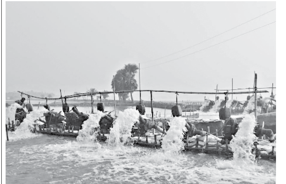
Water pumps are used to flush out the water from the fields in Bhabadaha area of Jashore's Abhaynagar upazila.
