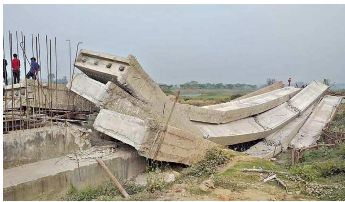
Five girders of an under construction bridge on Pagla-Jagannathpur-Raniganj-Aushkandi regional highway in Sunamganj's Jagannathpur upazila collapsed Sunday night. Officials of the construction company, MM Builders and Engineers Ltd, claimed that the accident happened when a hydraulic jack broke during the installation of a girder on a pier. The Road Transport and Highways Division has formed a four-member committee to investigate the incident.
