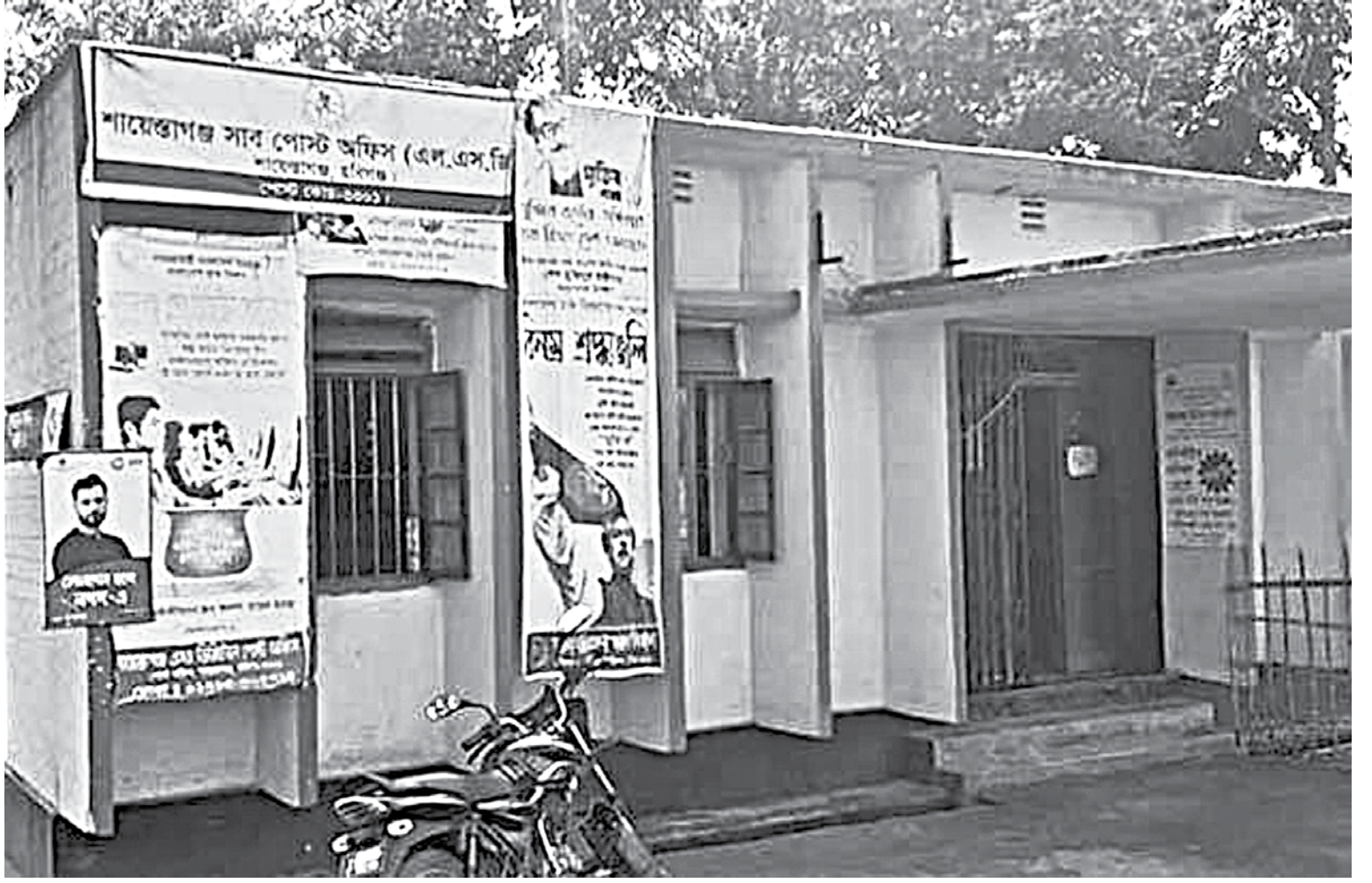
Shayestaganj post office building in Habiganj. Below, the building lies in a dilapidated state with plaster falling off ceiling.
