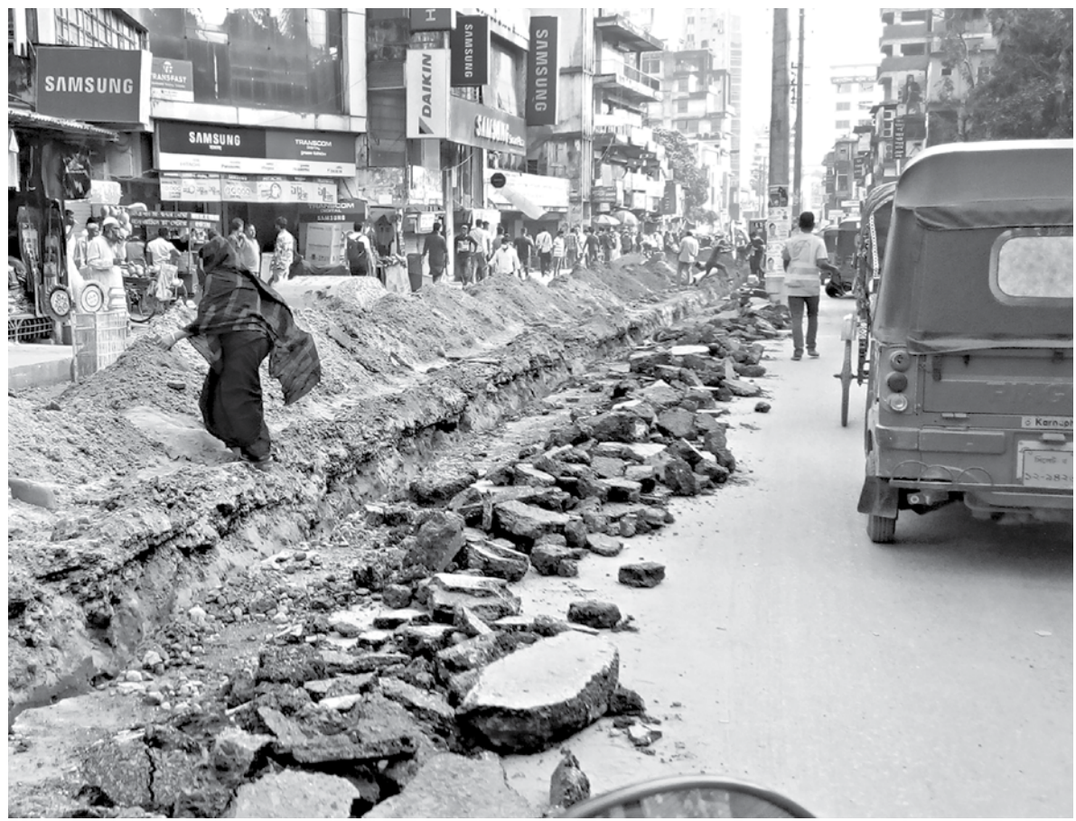
The main road of Sylhet city's Amborkhana area is dug almost down the middle for repair work on the area's water supply. This is taking its toll on pedestrians, vehicular movement, as well as on the busy area's entrepreneurs. Locals say their day-to-day activities would be far less disrupted if the development work was carried out from 8pm-6am instead of daytime. This photo was taken on Sunday.
