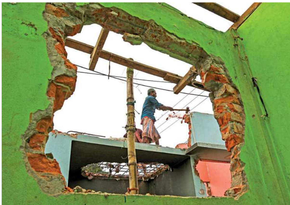
Walls of the many homes at Laldiarchar are being broken down, as residents of the area have decided to leave their houses ahead of a scheduled eviction drive by Chattogram Port Authority. Observing the situation, authorities chose not to use force to evict them. This photo was taken yesterday.
