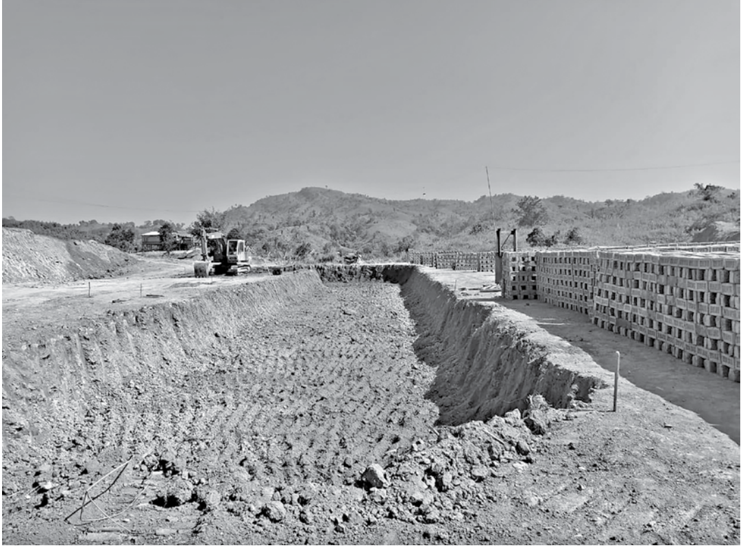
An excavator removes earth from beside the brick kiln that was built after felling trees and levelling hillocks at Romana Para of Bandarban's Ruma upazila. PHOTO: COLLECTED
